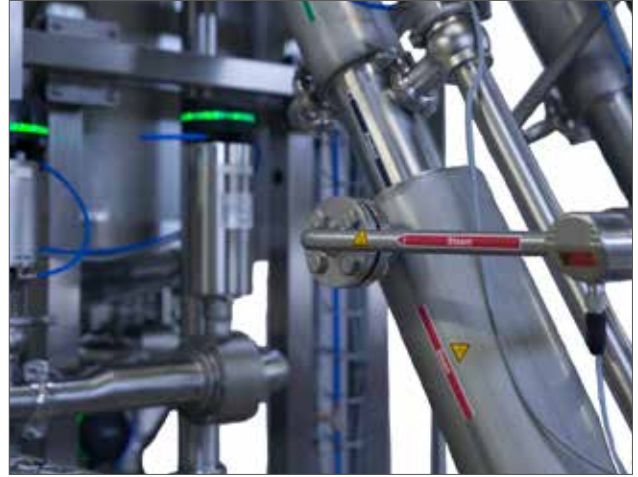
Steam jacket on salt auger.
